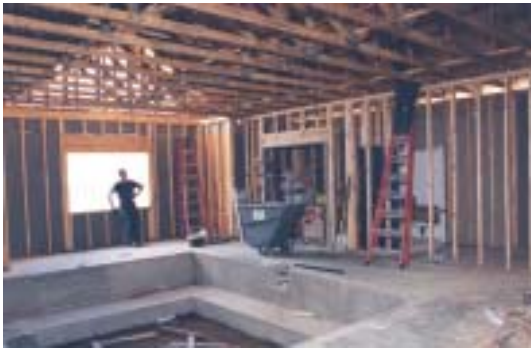
Warm water therapy pool under construction—one of the amenities in Kendal at Lexington's new health center.
